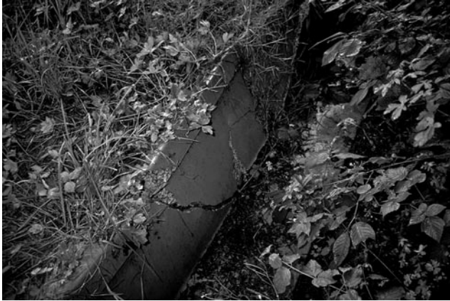
Fig. 3. Photograph of poorly maintained barrier wall. Some elements of the barrier wall are broken and overgrown by plants. Photograph by Silvia Zumbach.
