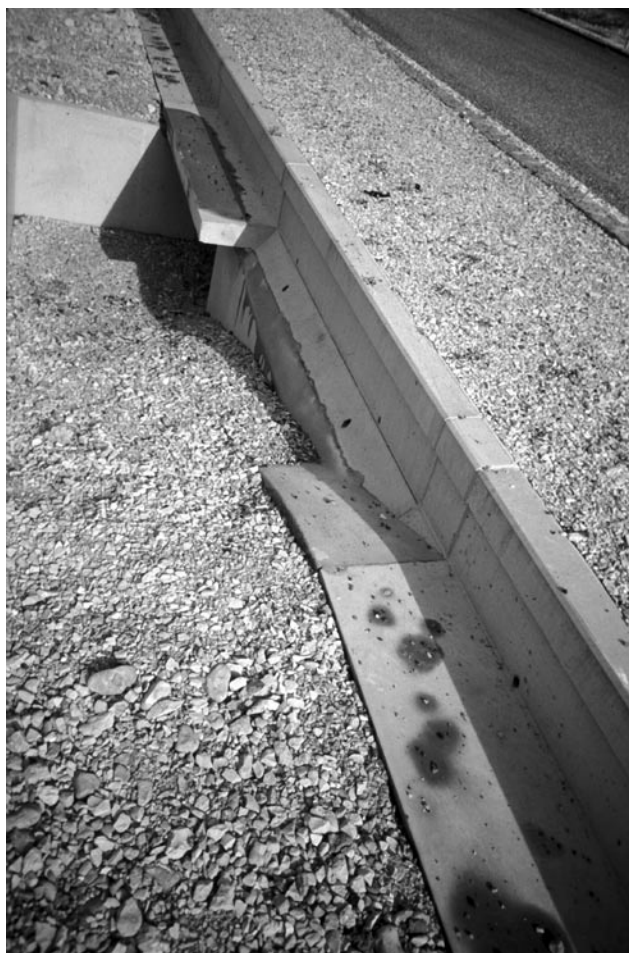
Fig. 2. Photograph of an underpass and barrier wall system near Porrentruy, Switzerland. The picture shows a concrete barrier wall, parallel to the road, made of L-shaped elements and the entry to a rectangular tunnel. Note (i) the walking surface along the barrier wall and (ii) that the upper end of the barrier wall is ground level with the surface of the road. The photograph was taken shortly after construction. Photograph by Silvia Zumbach
